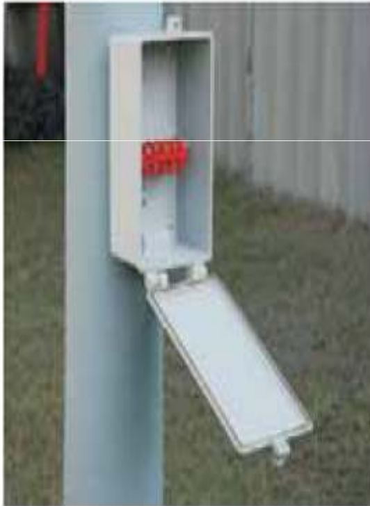
External Junction Box
