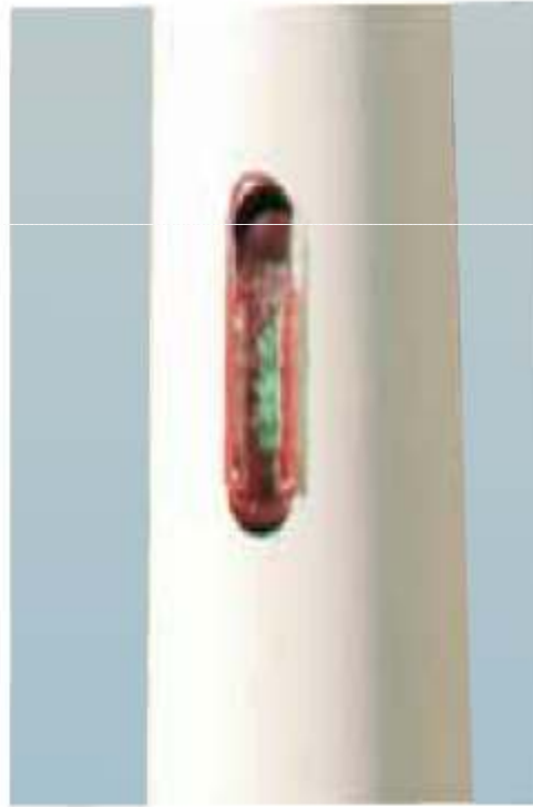
Internal Junction Box
