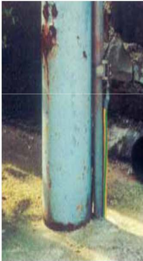
Rusted steel pole with required grounding
