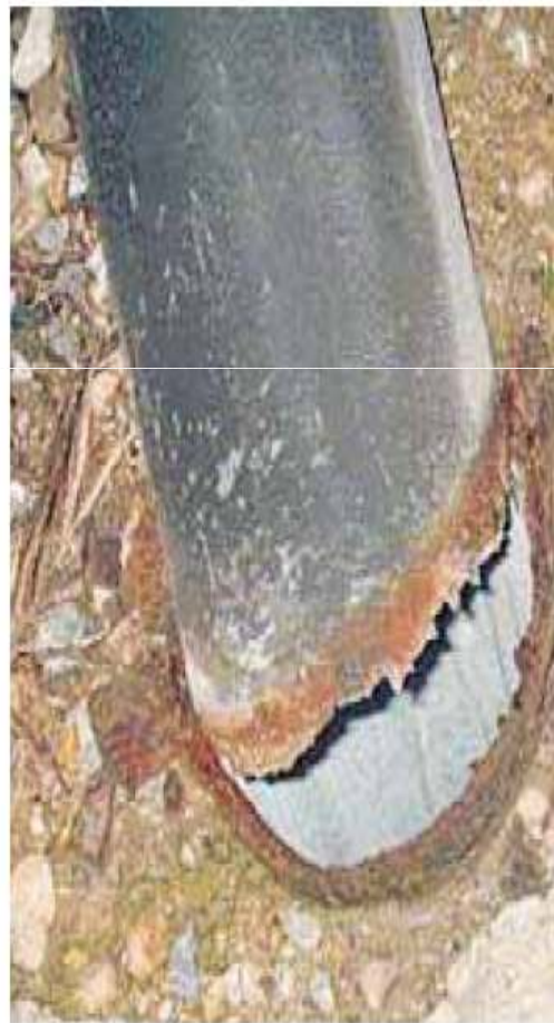
Weak Base of Steel Pole
